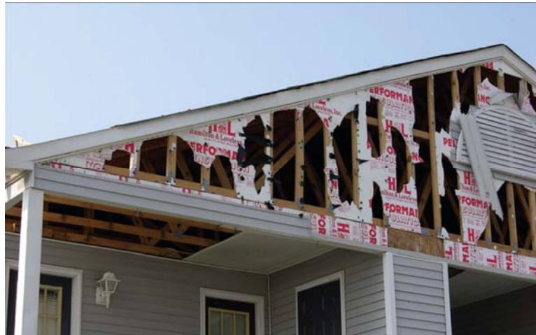
Fig. 2.15. PHOTO: Damage as a result of pressure differences. (FEMA 549 2006)
