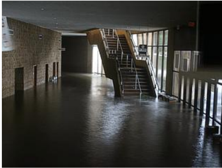
Fig. 2.3. PHOTO: Failure due to hydrostatic forces. (Collura, 2005)
