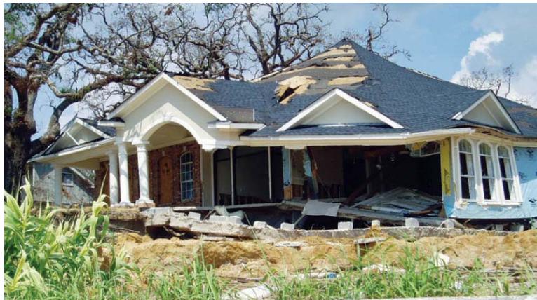
Fig. 2.4. PHOTO: Failure due to hydrodynamic forces. (FEMA 549 2006)
