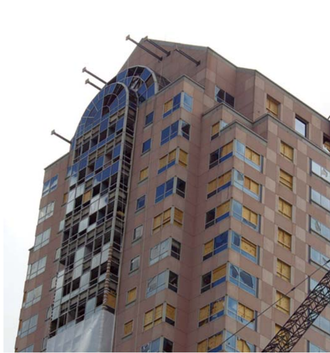
Fig. 2.16. PHOTO: Damage as a result of missile impact. (FEMA 549 2006)
